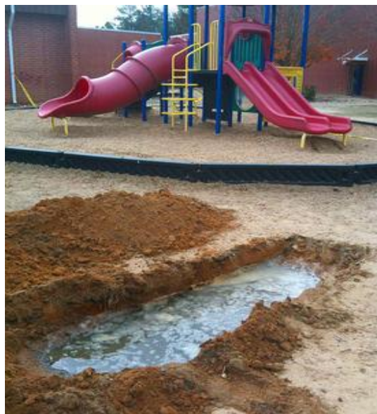
Failed septic system on a playground.
